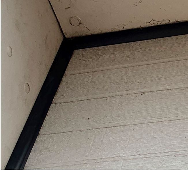
Figure B10: Sectional Door Exterior Jamb and Header Seals – Good Condition
