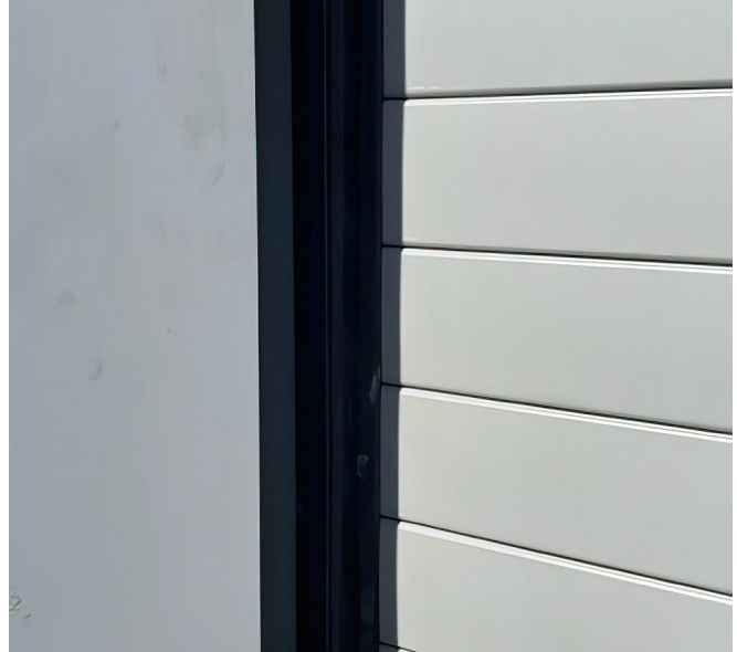
Figure B11: Rolling Door Exterior Guide Seals – Good Condition
