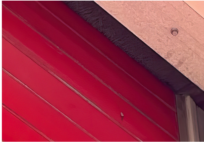
Figure B13: Rolling Door Exterior Jamb and Header Seal – Good Condition (Also see Figure B10)
