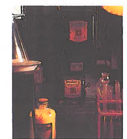
Square D safety switches in Edison's Fort Myers, Florida, research laboratory.
